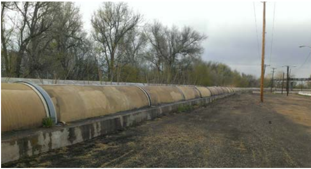
The Delgany Interceptor sanitary sewer lines run for almost 25 miles and are above ground along the NWC river frontage, creating a barrier between the NWC and the South Platte River.
